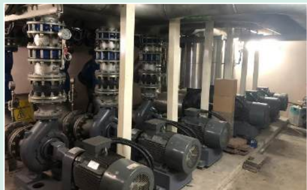
Existing cooling system
