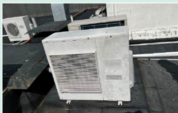
Installed condensing unit (On-site)
