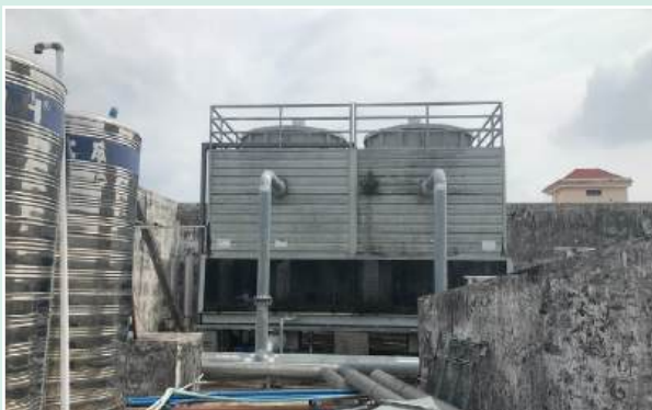
Rooftop condensing unit
