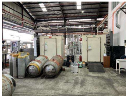
Reclamation facility (Malaysia)
