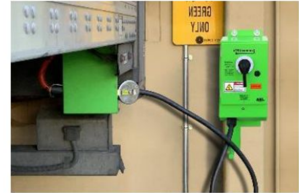
Shore Power – “Smart Power” Grid Powered Refrigeration
